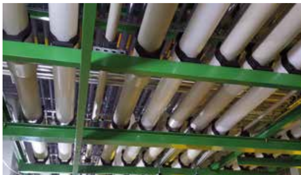
Figure B.3: PP piping system installed with AGRU pipe clips.
